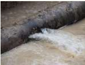
Leaking Pipes On Roads (Non Environment Friendly)
